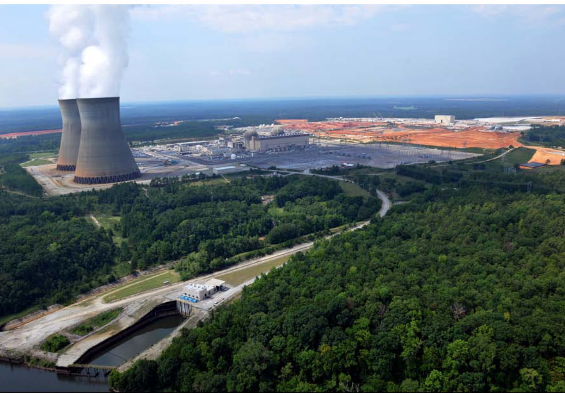
Aerial photograph of Vogtle site, with Vogtle 1 and 2 operating units to the left and Vogtle 3 and 4 construction site to the right. August 11, 2011
