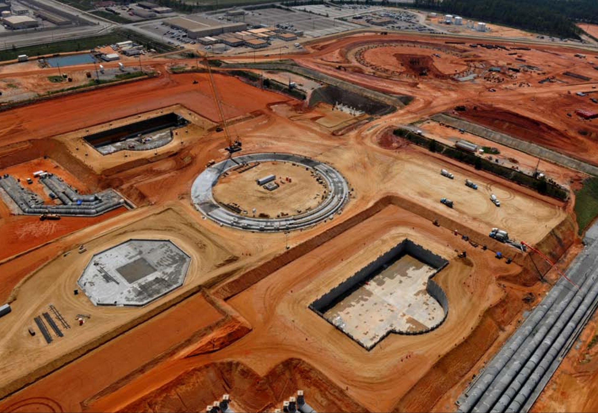
Aerial photograph of Vogtle 3 and 4 construction site. Unit 3 is located at left and top of photo and Unit 4 to the right and bottom. Heavy lift derrick crane foundation in center. August 11, 2011
