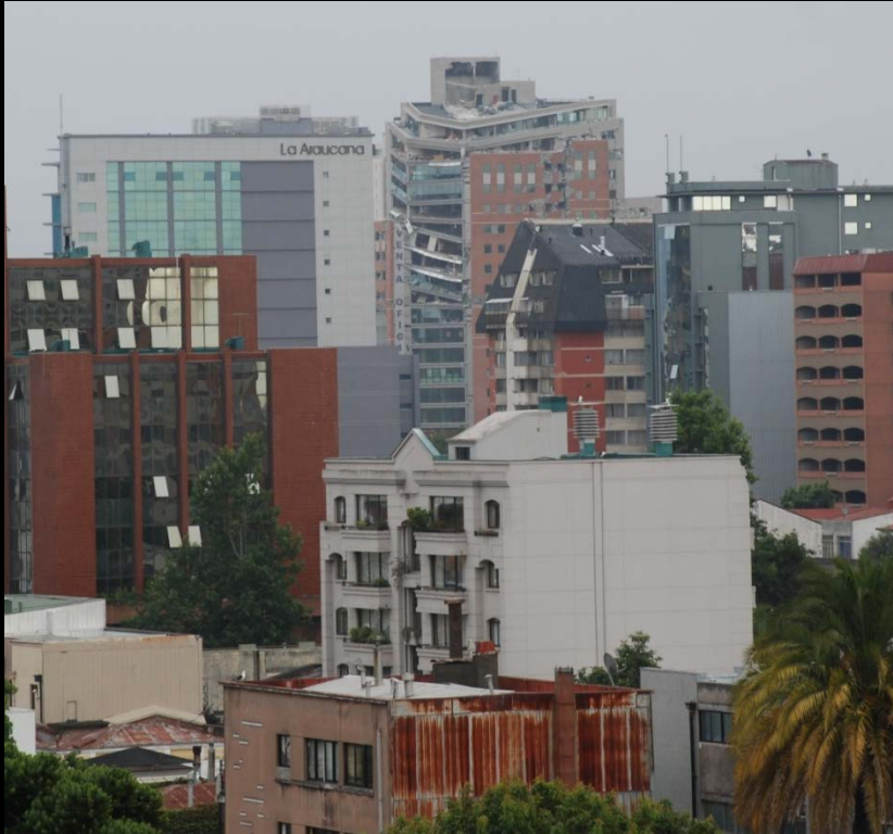
Partial collapse of 21-story O'Higgins building, tallest in Concepcion, threatens the surrounding built environment. Courtesy of J. Restrepo.
