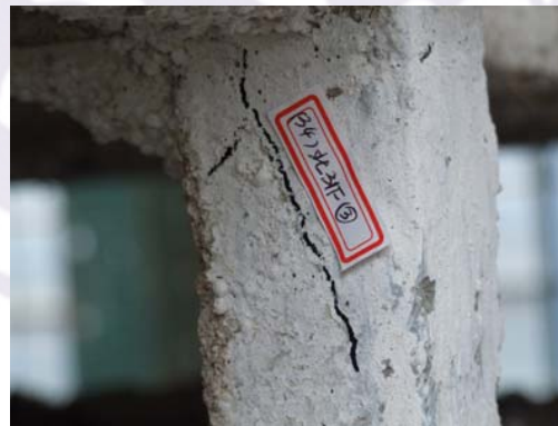
column diagonal crack in the 31st storey
