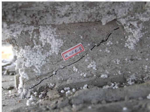
shear wall diagonal crack in the 30th storey
