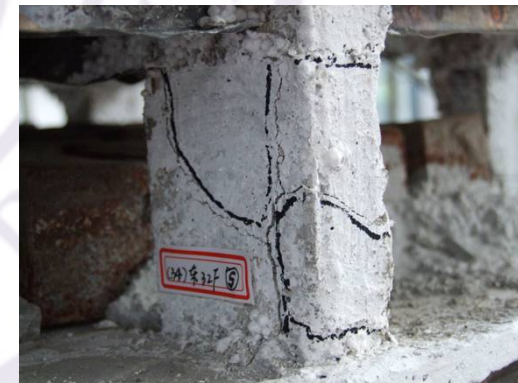
column crossing crack in the 32nd storey
