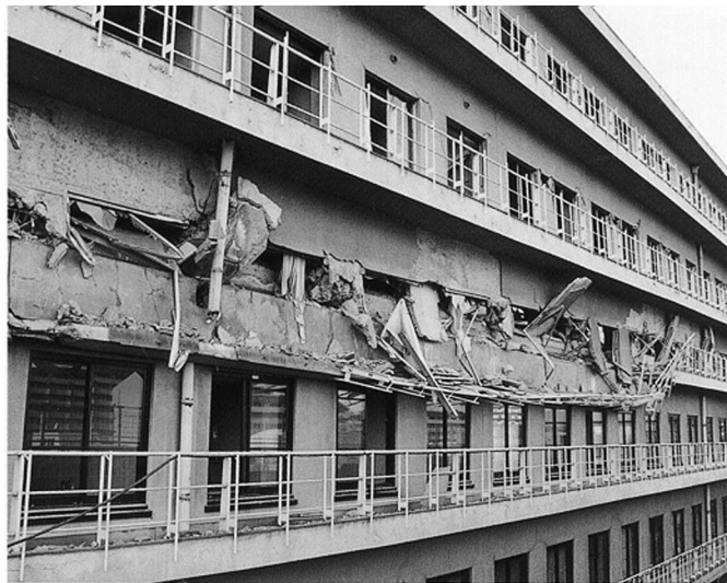
Figure 3 Gravity load collapse from 1995 Kobe Earthquake (AIJ, 1997)
