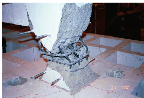
b) North short column failure (B2)
