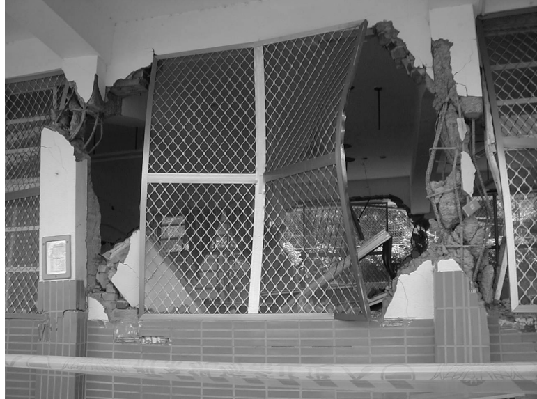
Figure 2 Apparent loss of column axial load capacity without collapse of building frame from 1999 Chi-Chi Earthquake
