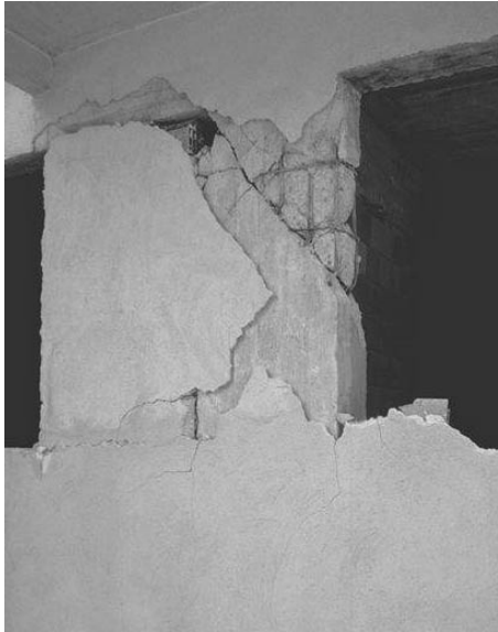
Figure 1 Column shear failure from 1999 Kocaeli Earthquake
