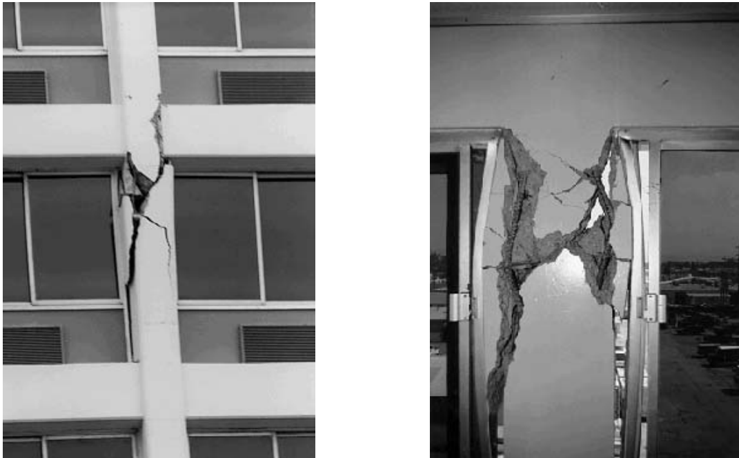
Fig. 3.3 Examples of structural damage in the building due to 1994 Northridge earthquake; shear failure of columns in the south face at fifth story. [After Naeim 1997].
