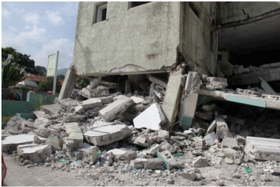
Fig. 17 Collapsed building in Haiti.
