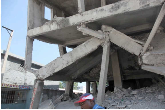
Fig. 13 Damaged first-level of a building in Haiti.
