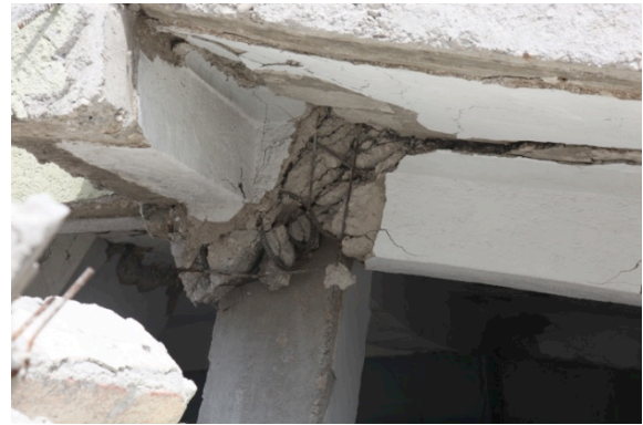
Fig. 16 Close-up of collapsed building.
