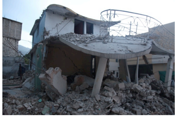
Fig. 14 Damaged house in Haiti.
