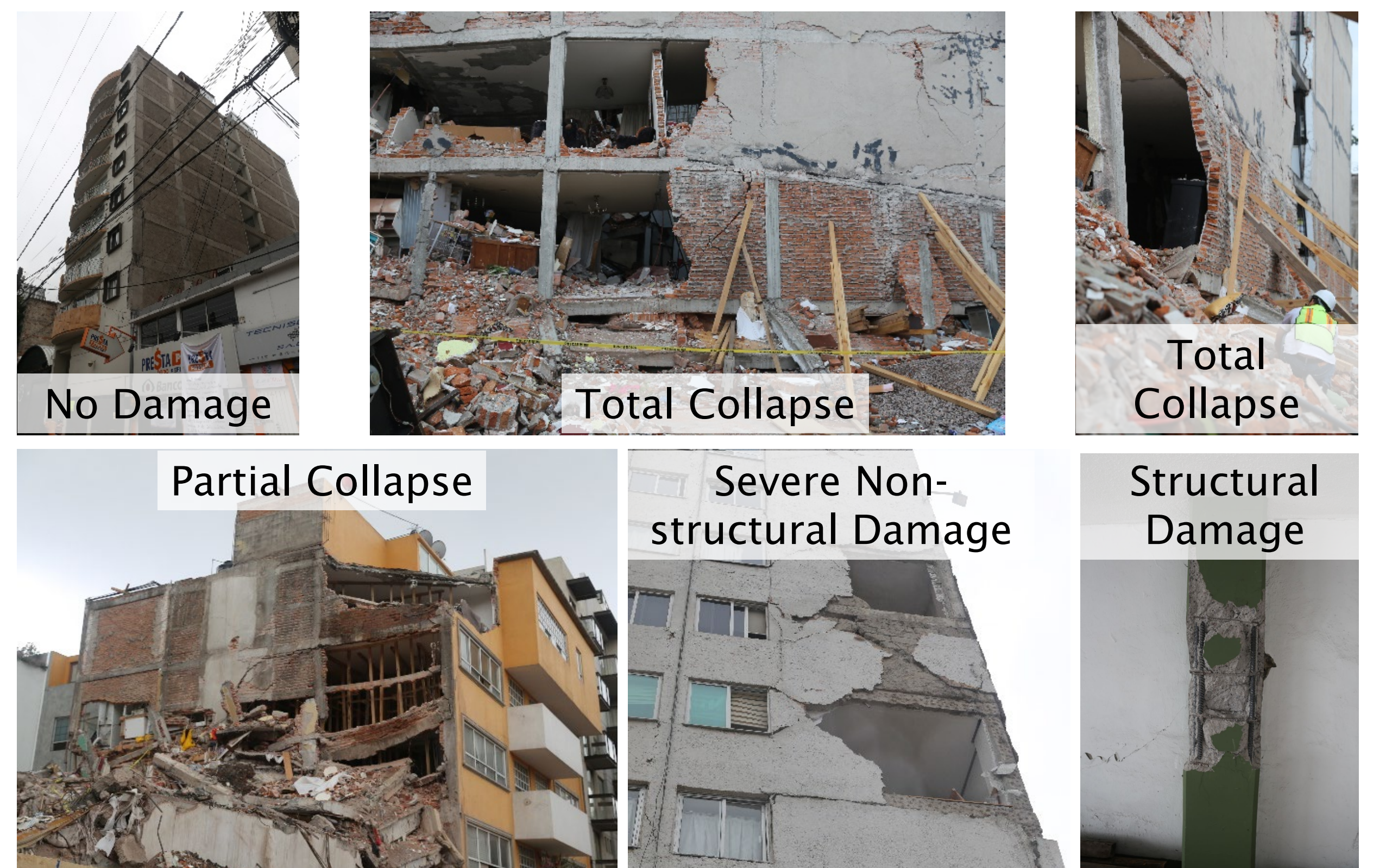
Figure 2. Examples of observed damages.
