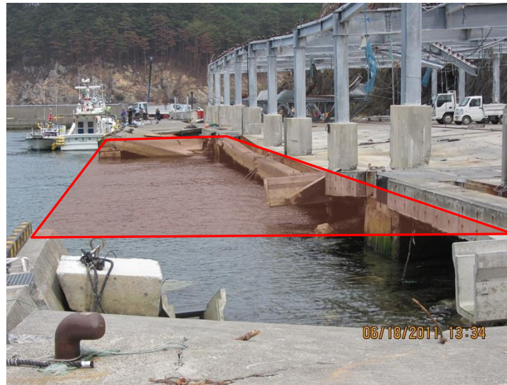
Damage to the Omoe Fishing Port, Omoe. Credits: H. Yeh
