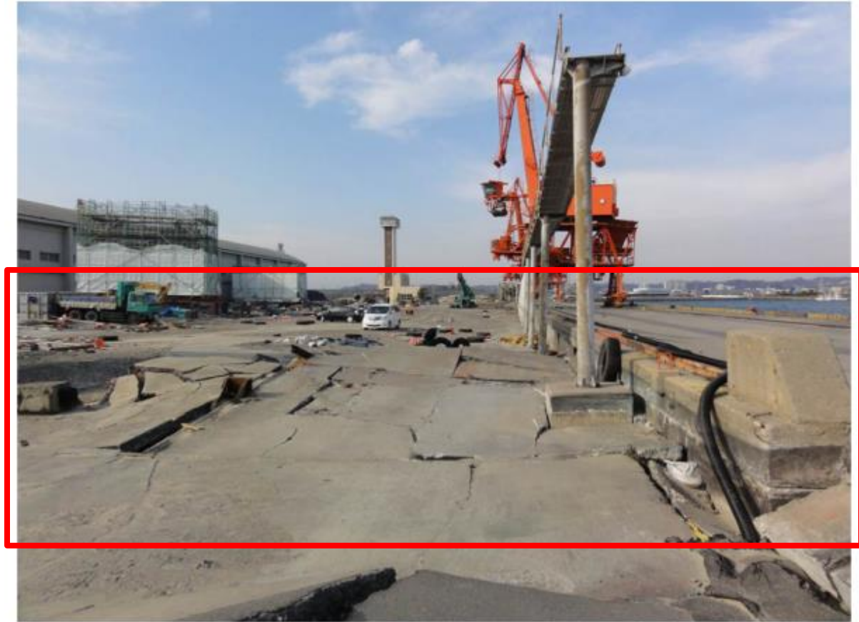
Damage to the 10 m deep Berth 3-2 in the Third Wharf Area of Onahama Port. Sugano et al (2014)
