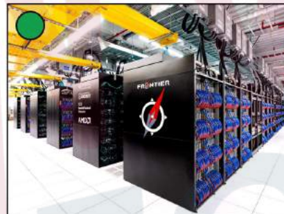
Frontier (completed 2023) Oak Ridge National Lab Oak Ridge Leadership Computing Facility (OLCF) 9402 GPU accelerated nodes 4 AMD MI250X GPUs / node 1.194 ExaFlops Top500.org #1
