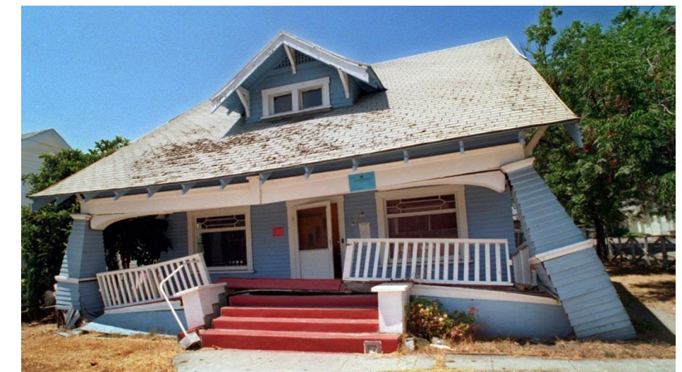
Life Safety Level of Damage for an Ordinary Building after a Large Earthquake
