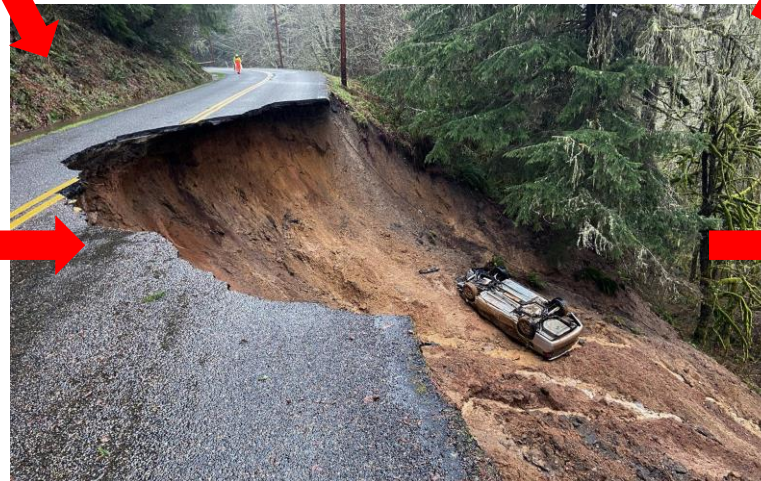
Southern California Landslides (2024)
