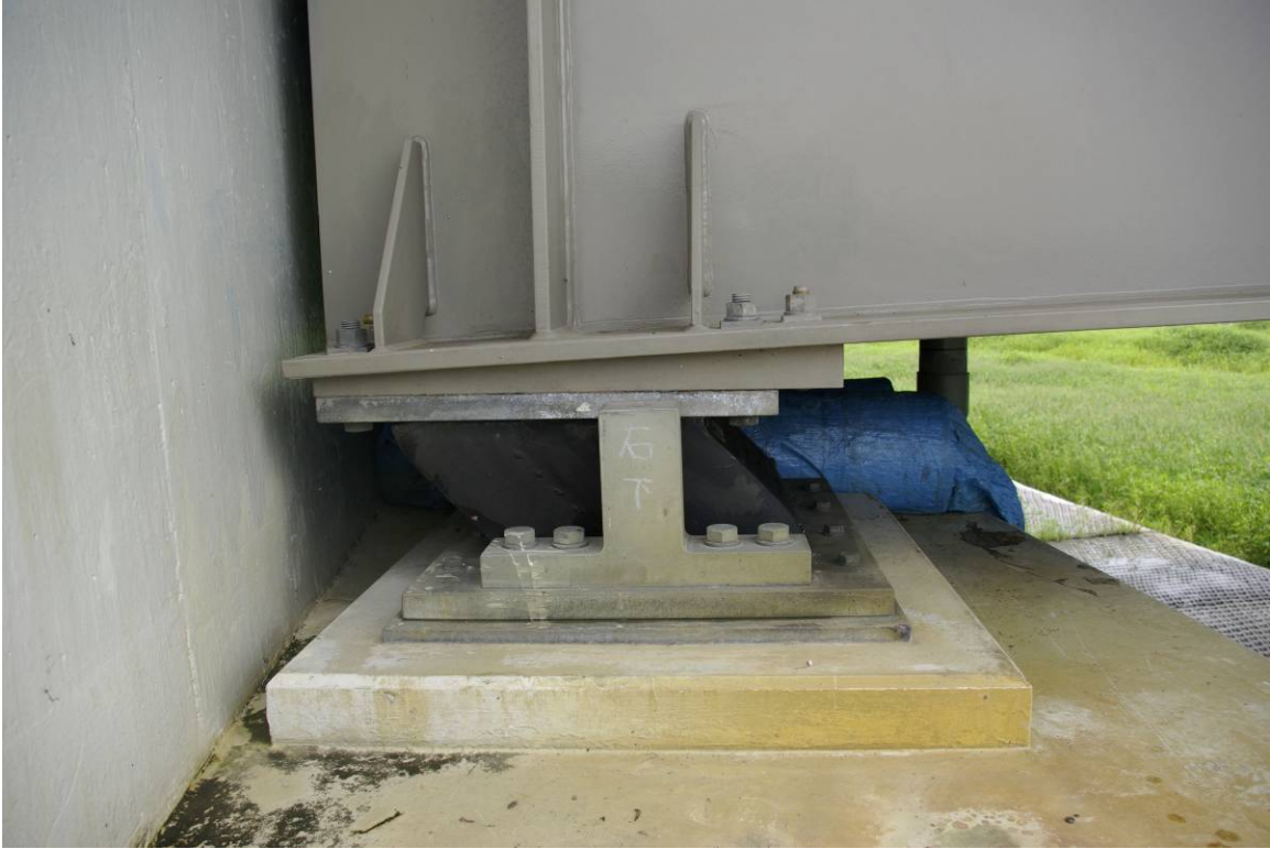
Figure 1.11 Permanent offset in elastomeric bearing at Nagomi Bridge caused by ground deformation during the Niigata Chuetsu-Oki earthquake (Kayen et al. 2007).
