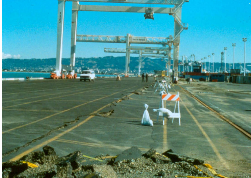
Figure 1.2 Top of the wharf of Port of Oakland following the 1989 Loma Prieta earthquake. The cranes separated and could not operate as a result of the extension of the wharf (photo by John Egan, AMEC).
