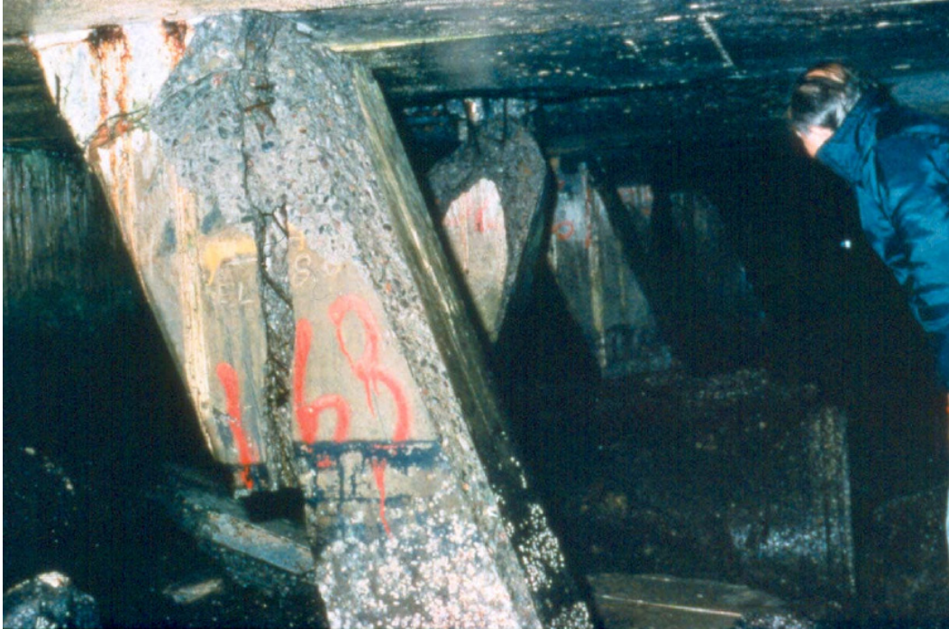
Figure 1.4 Damage to the battered piles supporting the wharf at the Port of Oakland during the 1989 Loma Prieta earthquake (photo by John Egan, AMEC).
