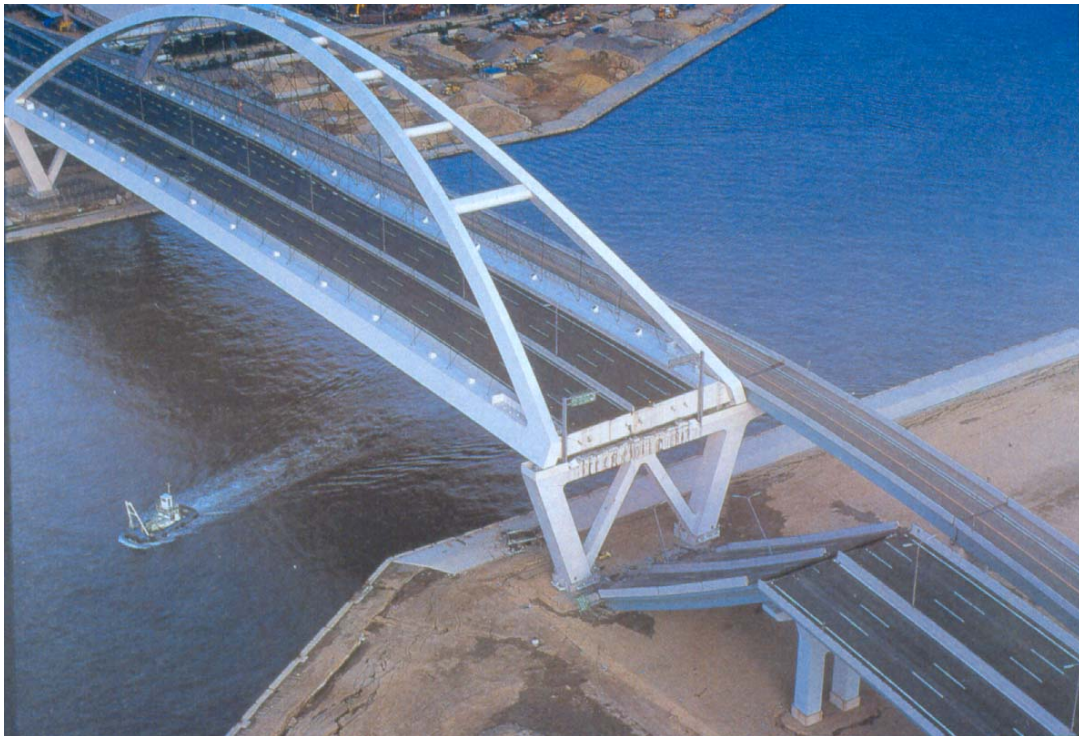
Figure 1.5 Unseating of the Nishinomiya Bridge as a result of lateral spreading during the 1995 Kobe earthquake.
