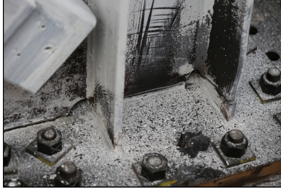
Figure 5.41 Fracture at the west column base.
