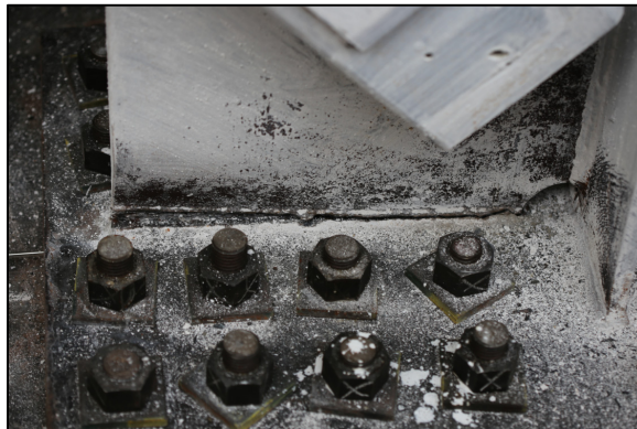
Figure 5.40 Fracture at the west gusset-to-baseplate weld.
