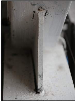
Figure 5.36 Fracture at the second-story west gusset-to-beam weld.
