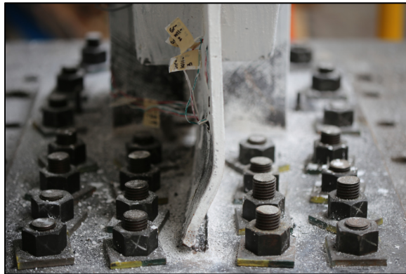
Figure 5.39 Fracture at the west gusset-to-baseplate weld.
