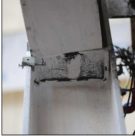
Figure 5.27 Twisting of first-floor beam at east connection after shear tab tear.
