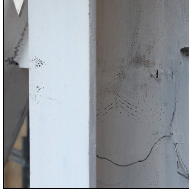
Figure 5.65 Whitewash flaking behind weak-axis west column at roof gusset plate.
