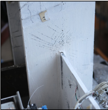
Figure 5.16 Typical flaking near the tip of the gusset plates.
