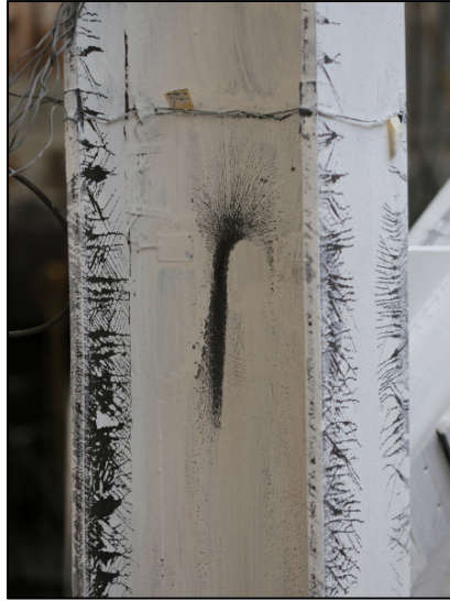
Figure 5.30 Yielding of east-column web near the column base behind first-story lower gusset plate.
