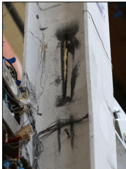
Figure 5.31 Tearing of east-column web behind the second-story lower gusset plate.
