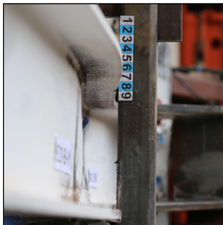
Figure 5.29 Curvature and final downward displacement of the first-floor beam.
