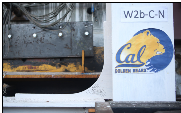
Figure 5.64 Whitewash flaking at west first-floor gusset (potentially left from original frame before strongback “retrofit”).
