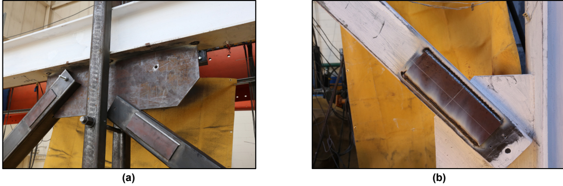
Figure 3.7 Repair of second story of NCBF-B-1: (a) erection of braces; and (b) added net-section reinforcement.
