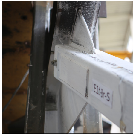
Figure 5.28 Weld fracture at the first-story center gusset.
