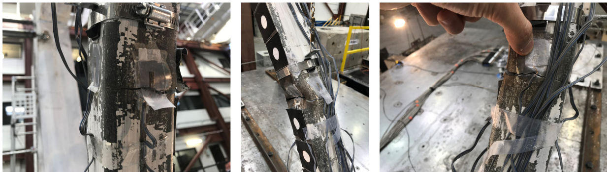
Figure 5.25 Specimen 2 ruptured braces locations.
