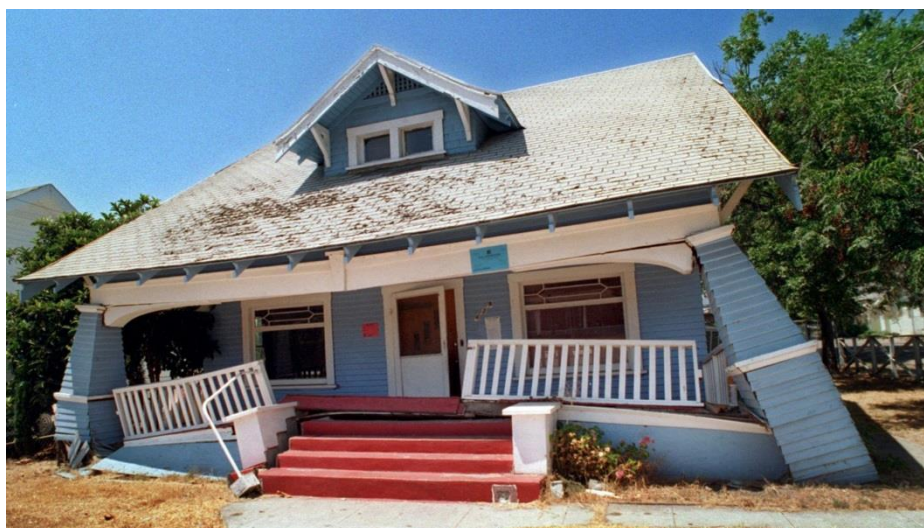
Life Safety Level of Damage for an Ordinary Building after a Large Earthquake
