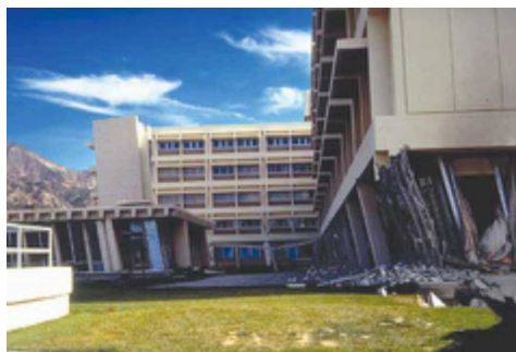
Figure 3.2: Iconic soft-story failure of Olive View Hospital during 1971 San Fernando, California earthquake. (Image courtesy of the USGS).
