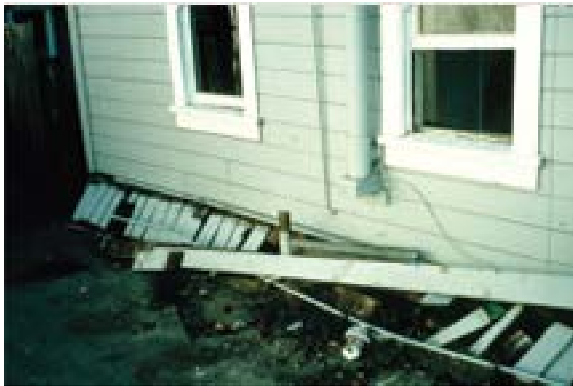
Figure 1. Typical cripple wall failure (SPUR, 2012)
