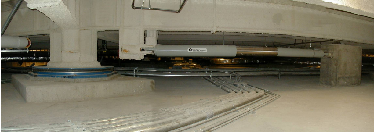
Figure 2.3: Supplemental viscous damper at isolation plane to control displacement (New de Young Museum, San Francisco, CA, courtesy of Rutherford & Chekene)
