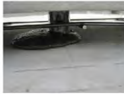
(f) Overflow of grout from coupler
